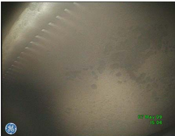
Figure 4: Typical Stage-1 Thermal Barrier Coating (TBC) blade after 21,650 hours of operation
