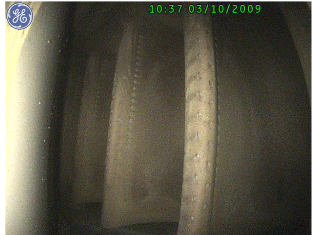
Figure 1: Typical Stage-1 blade after 5,000 (new)/12,200 (refurbished) hours of operation
